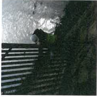
A Extended fence down revetment
